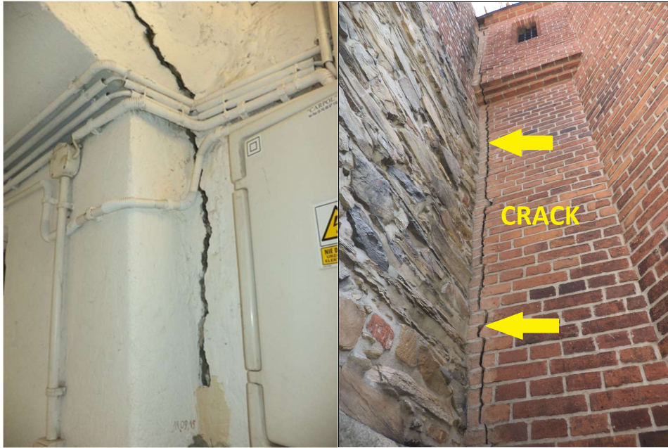
Fig. 3. Crack at the connection of the tower and the outbuilding – the view from inside and outside
